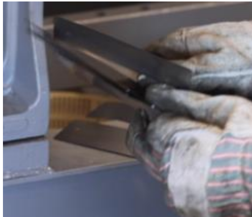
Figure 4-126: Add More Shims to Shim Pack To Achieve Required Indicator Reading
