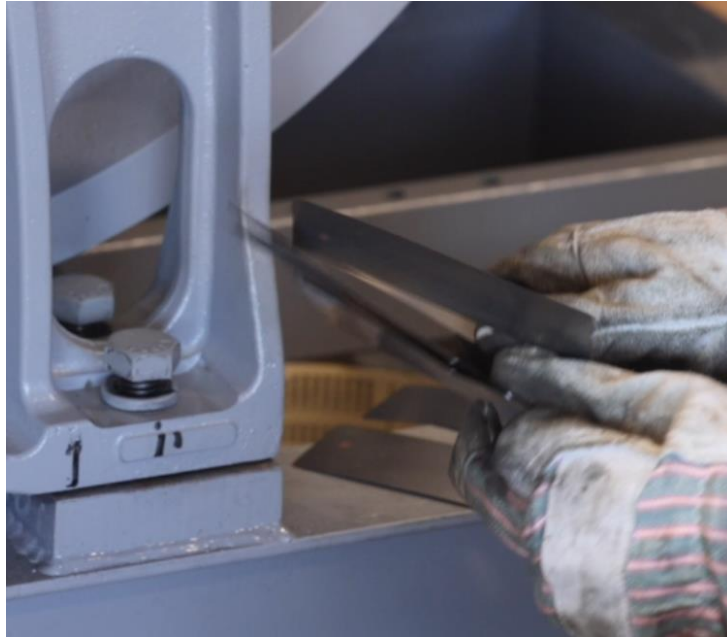
Figure 4-107: Add More Shims to Shim Pack To Achieve Required Indicator Reading
